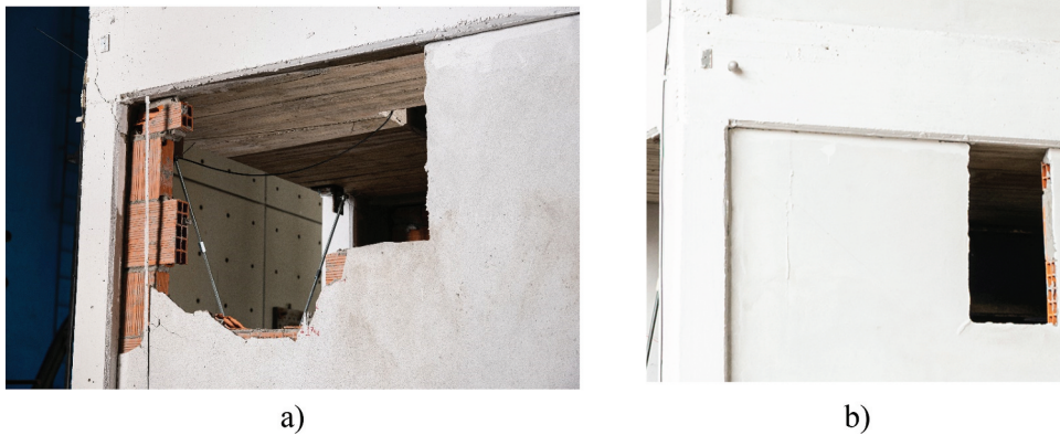
Figure 12. Detailed view of a selected region of the Buildings: a) cracking of the column-slab joint region of the first floor in Building A, b) column-joint region of Building B with no signs of distress.
